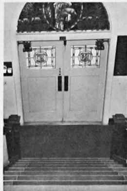
Steps dangerous for young and old.
